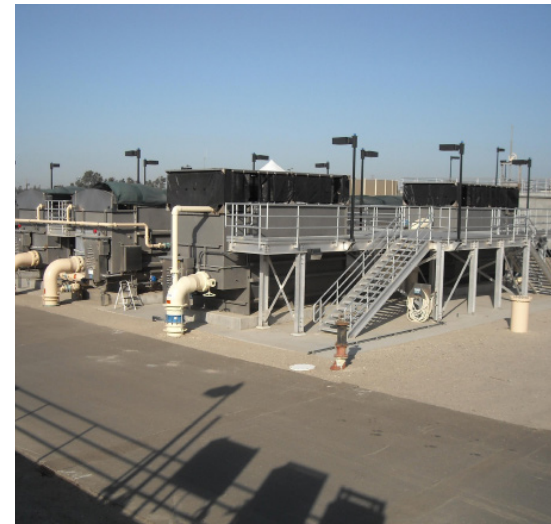
Tertiary Filters at the RWQCF help treat the water to a very high level, allowing it to be used in the community for landscape irrigation, for agricultural irrigation, for cooling water, or other nonpotable uses.
