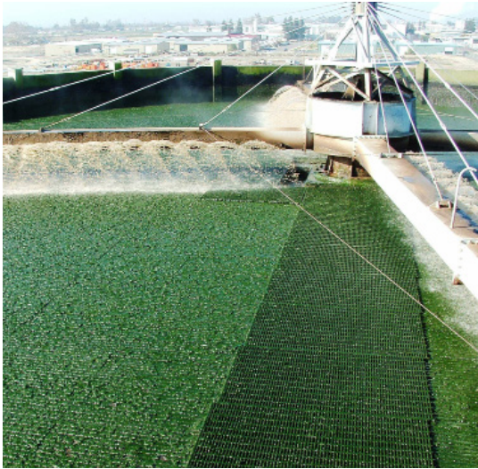
The RWQCF, last upgraded in 2006, treats wastewater from Turlock and the neighboring communities of Keyes and Denair.
